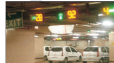
NDMC Parking Guidance Systems
